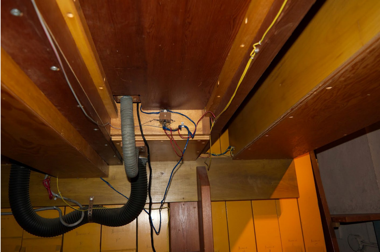
Figure 4: Poor-quality wiring underneath the Choir Organ chest.
